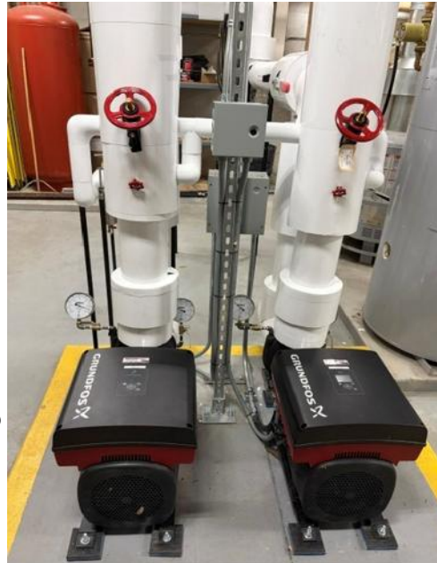
MSS Chiller Pumps
